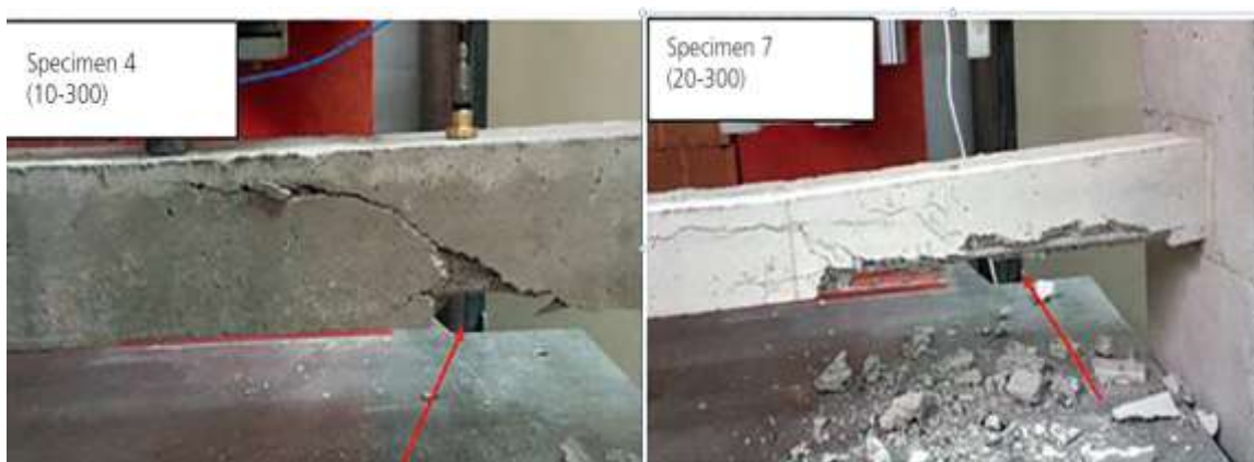
Fig. 17. Crack distribution of the samples [17]
