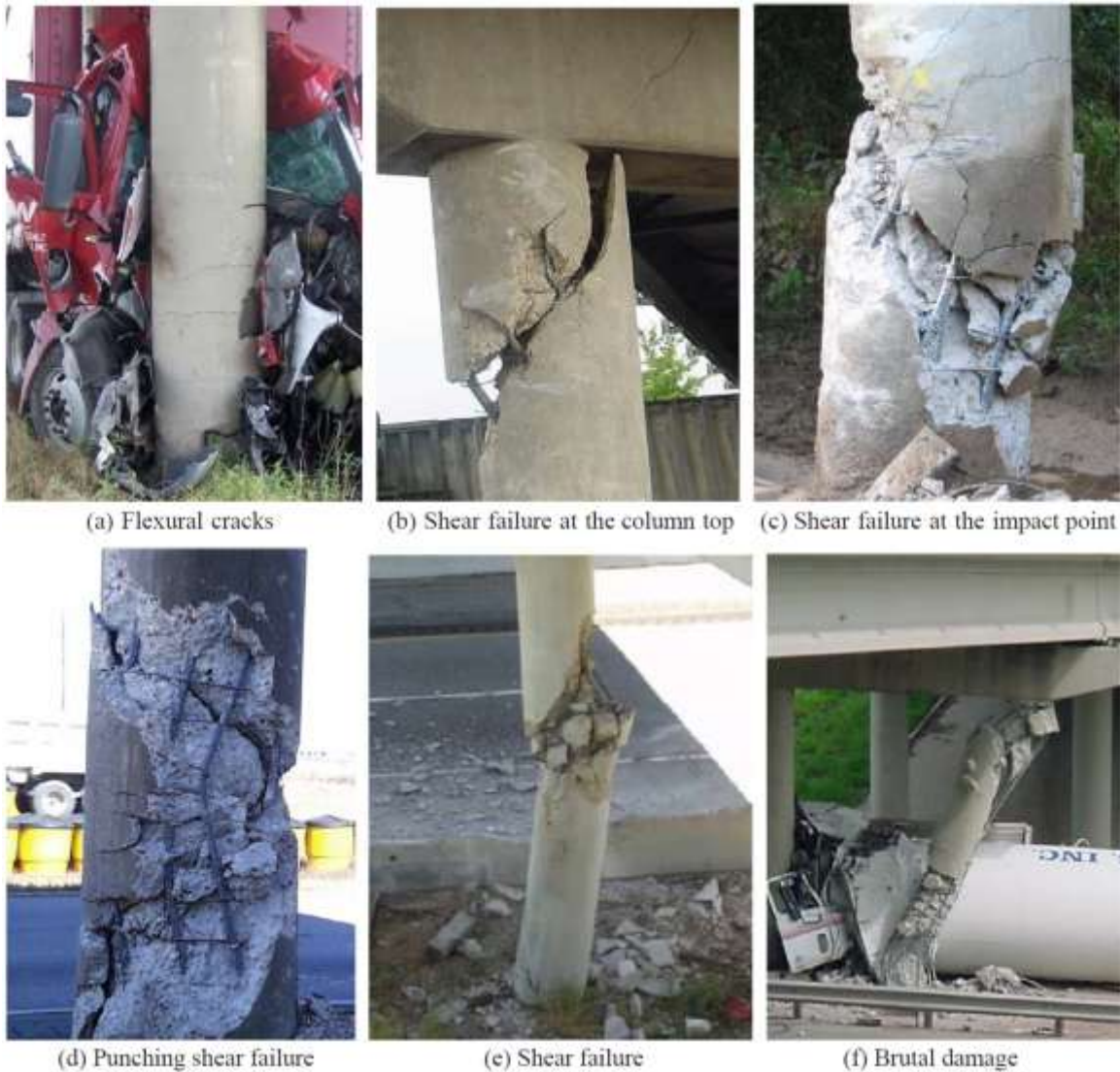
Fig.3. Failure mode of bridge columns [12]
